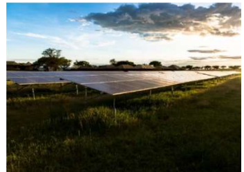
Example 2: Off-Grid system for tourist resort in Tanzania with 130 kWp and 900 kWh lead-acid battery storage.
