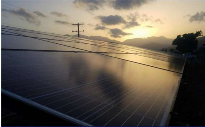
Figure 2 - Operating Mini grid in Haiti (Courtesy of Earthspark International)
