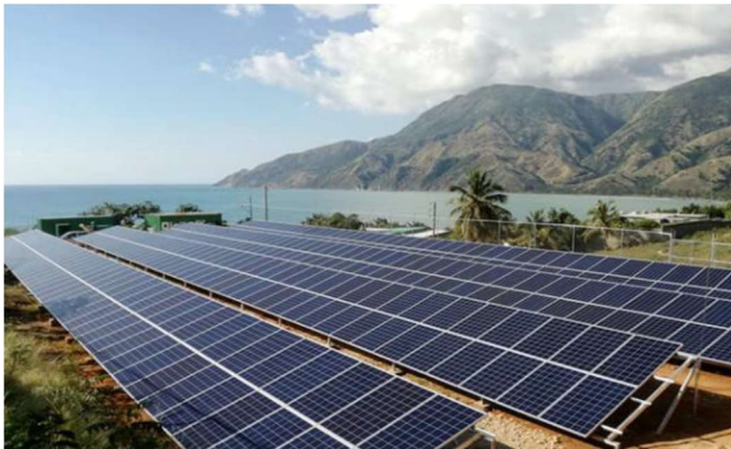
Figure 1 - Operating Mini grid in Haiti (Courtesy of Earthspark International)
